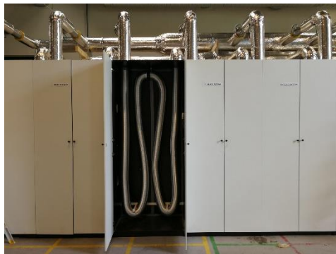
Figure 3-6. Cooling system integrated into the compartments in the laboratory hall.
