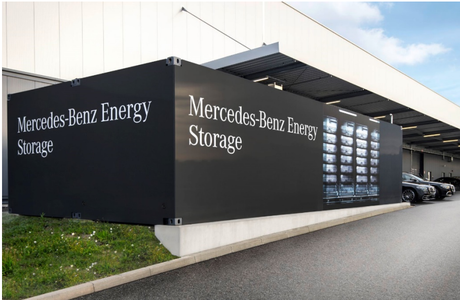
Figure 6. Second Life Battery Energy Storage at the Mercedes-Benz production site in Sindelfingen, Germany 7
