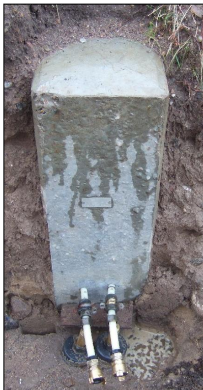
Figure 15: A single EP at the Langmarksvej test site prior to connecting the TRT equipment.
