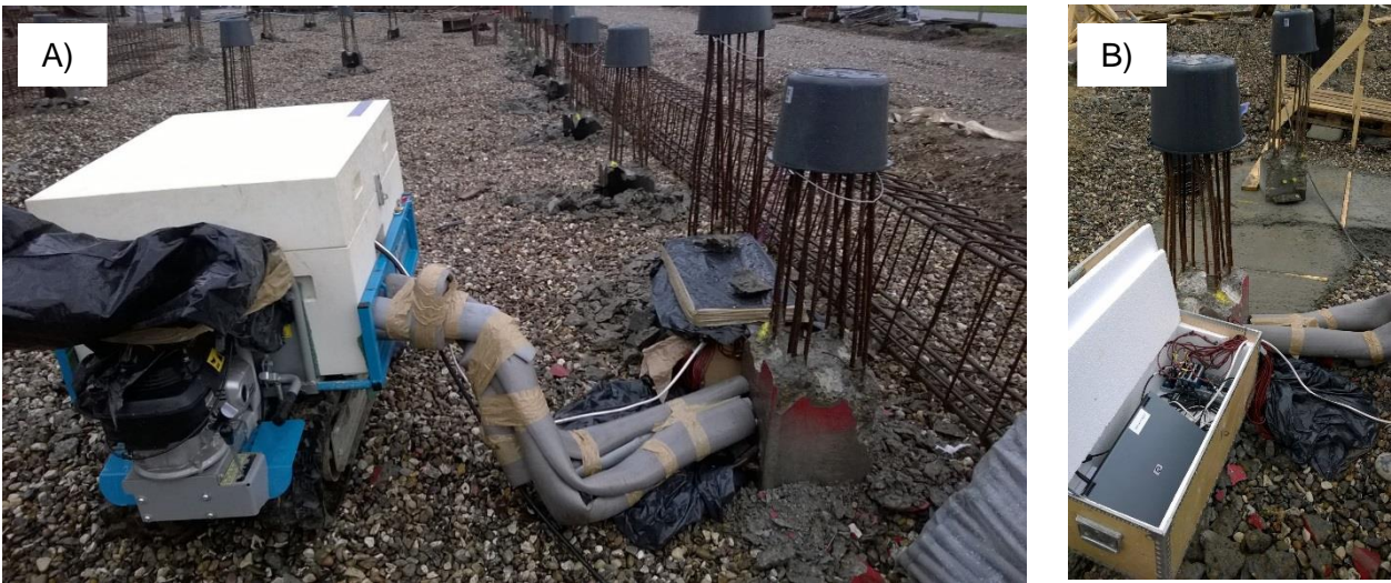
Figure 21: A) Ongoing TRT of the 16 m long EP at Rosborg North. Inlet- and outlet pipes are insulated to prevent disturbances from ambient conditions. B) The adjacent box, covered with black plastic bags contains the computer and the modules to log the temperature data from the Pt100 temperature sensors casted into the pile (see Figures 11 and 20).
