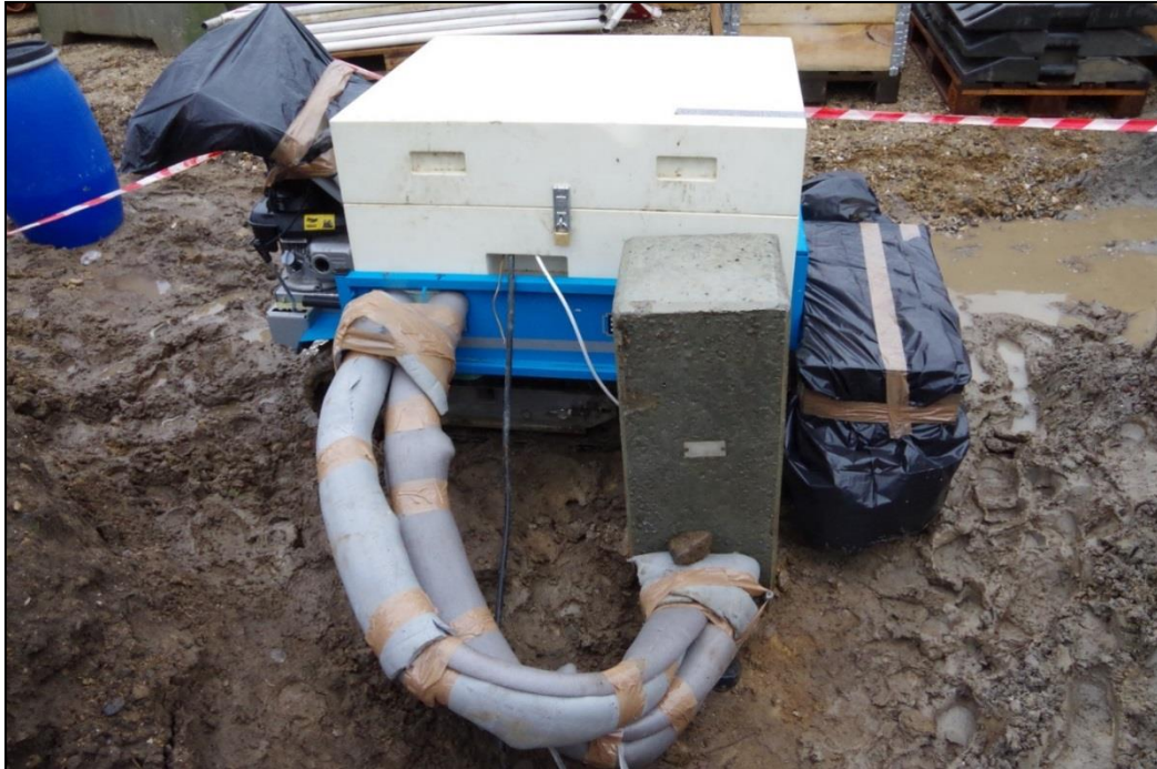
Figure 18: Ongoing TRT of the 18 m long EP3 at Langmarksvej. Inlet- and outlet pipes are insulated to prevent disturbances from ambient temperature conditions. The adjacent box, covered with black plastic bags, contains the computer and the modules to log the temperature data from the underground Pt100 TSA.
