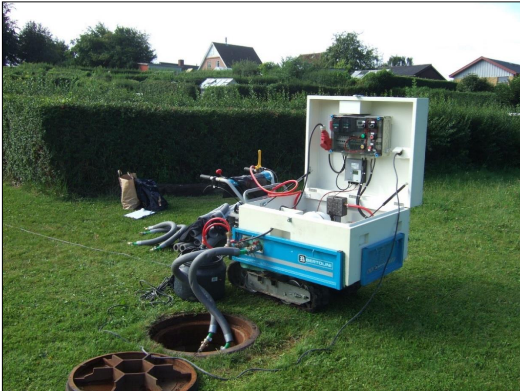
Figure 14: Ongoing TRT at the 18 m deep BHE at Langmarksvej. Inlet- and outlet pipes are insulated to prevent disturbances from ambient temperature conditions.
