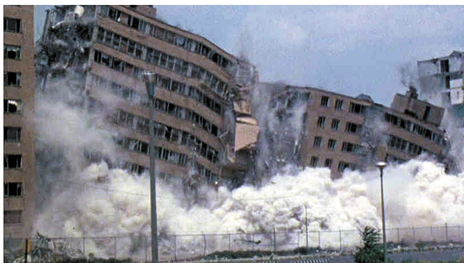
Figure 4.3 The 1972 demolition of the 'Pruitt-Igoe' social housing in St. Louis, USA, which Charles Jencks proclaimed as 'the end of modernism' epitomizes the failure of rational-comprehensive planning.
