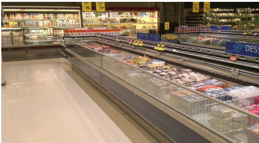
Figure 1.1: Supermarket display cases. Freezer gondolas are located in the front and open shelf type fridges are located in the back.
