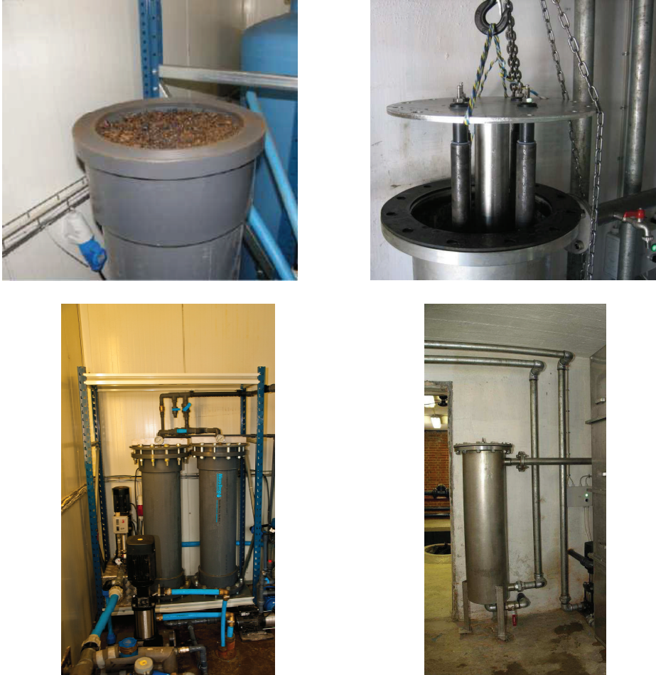
Figure 12 Danish waterworks, where the system is mounted with the ZVI capsule (pictures on the left) and the Fe-ED (on the right); the iron generator is connected to the aeration unit on the right lower picture (courtesy of MicroDrop Aqua ApS, Denmark)
