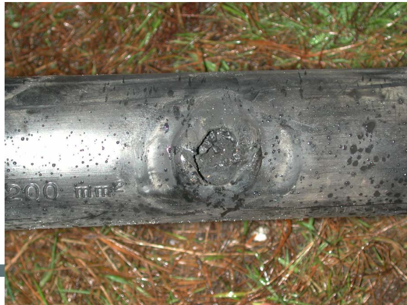
Photo of a single phase cable fault at the onshore part of the Horns Reef 2 170 kV HVAC cable. From PhD Thesis by Christian F. Jensen, 2013.
