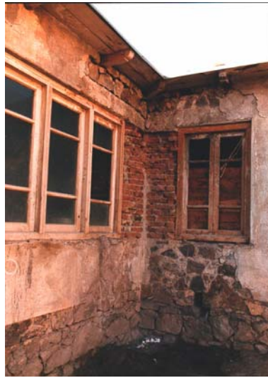
Fig. 436 Plaster finishing erosion
