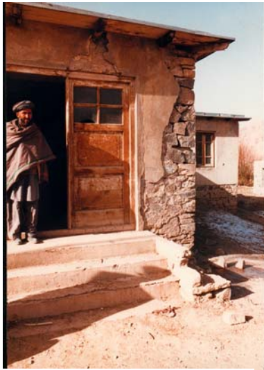
Fig. 435 Plaster finishing erosion
