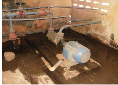
Pump, pumping the water from the dam to the filters
