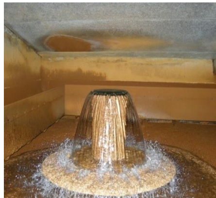
Fountain aeration process in Astrup WTP
