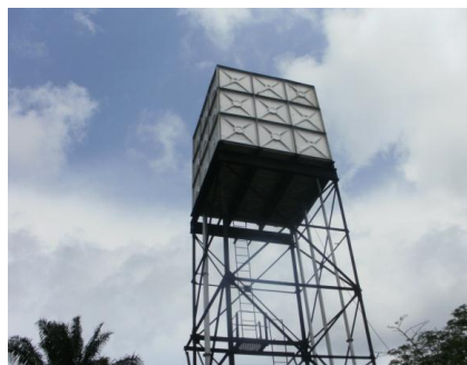
Water distribution tank
