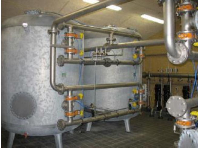
Figure 9.6: Picture of the model plants to be constructed in Ghana, exhibiting two filter vessels connected in series for double filtration.
