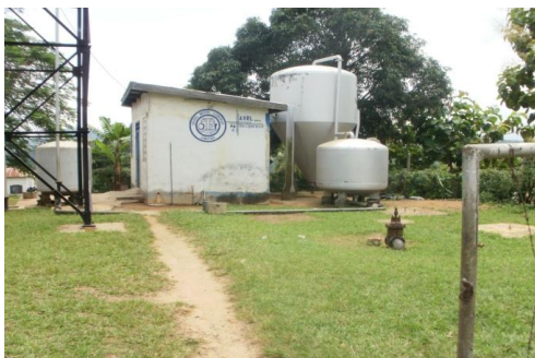
Sand filtration tank
