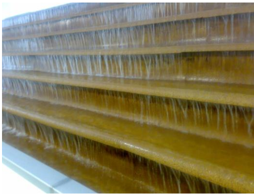
Cascading aeration method in Holstedbro WTP
