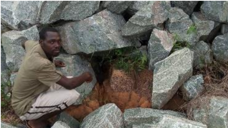
Figure 28 Alleged leakage from Tailings Storage Facilities (TSFs)
