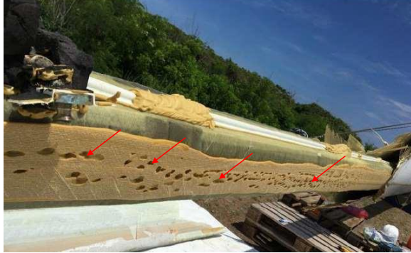
Fig. 1.12: Shell disbonding from box spar. The red arrows indicate where some of the voids are located in the adhesive layer. Adapted with permission from Find Møhlolt Jensen, Bladena.
