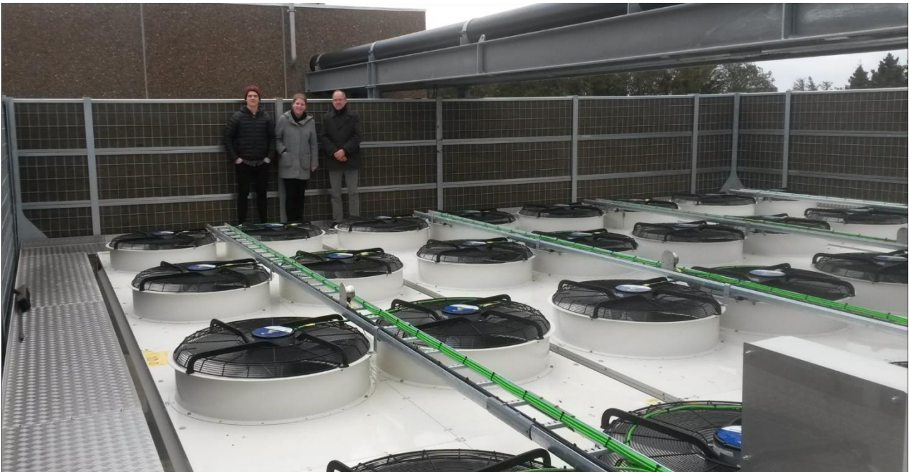
Figure 23: The ambient air heat source for the HP at Ringkøbing DE plant [119].
