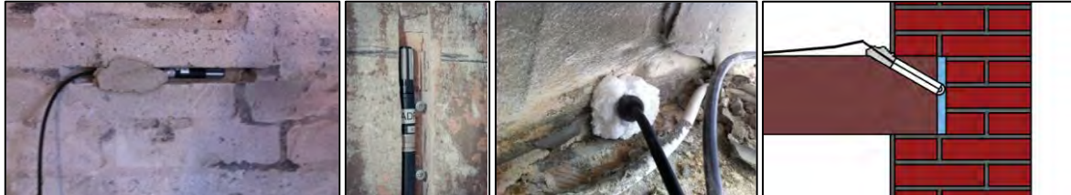
Figure 10: Sensor locations, left to right: in existing joint, in man-made notch in existing wall, and sealed in behind beam end [1].
