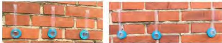
Figure 4: Karsten tube measurement on brick (left) and mortar joints (right). (Images from test building 2).
