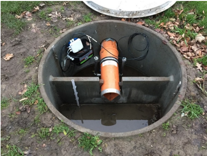
Figure 2.7. Flow-meter manhole with a V-notch weir.
