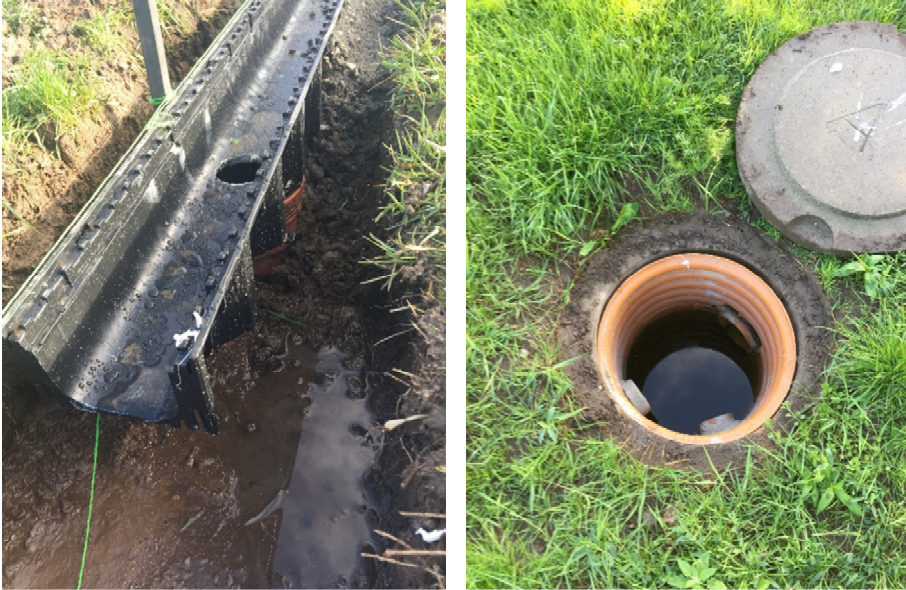
Figure 2.6. Left: Outlet from line drain to the grit chamber. Right: Grit chamber. Two inlets are seen at the bottom of the picture and one outlet towards the flow-meter at the top.
