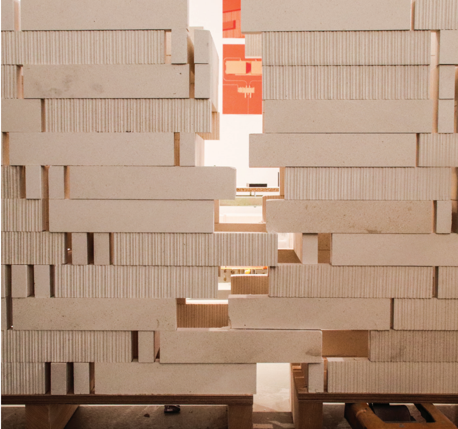
Figure 5.2. The limestone brick wall was produced as four separate sections. Here two of the sections are being joined together. Photo by Isak W. Foged.
