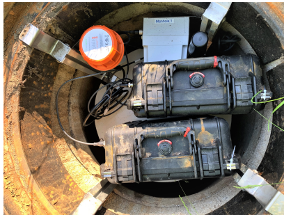
Figure 4.18: Level sensor deployed inside a manhole. The data in the Ishøj Case Study have been obtained through level sensors equipped with battery and wireless communication, sending data at every 2 minutes to our data base.
