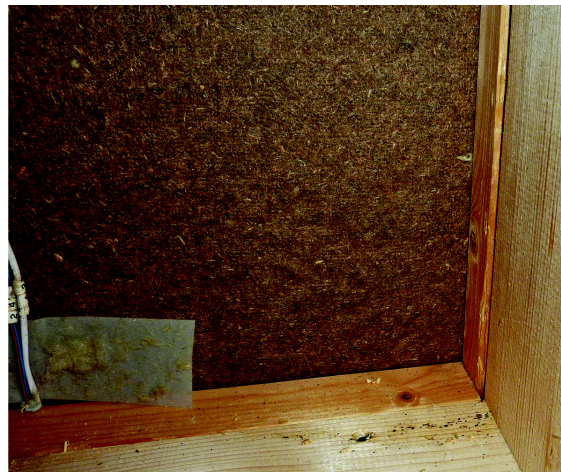
Figure 9 Inner side of the wind barrier after four years of exposure: element 14, facing north (vertical weatherboard, no cavity, wind barrier: asphalt-impregnated wood fiberboard).
