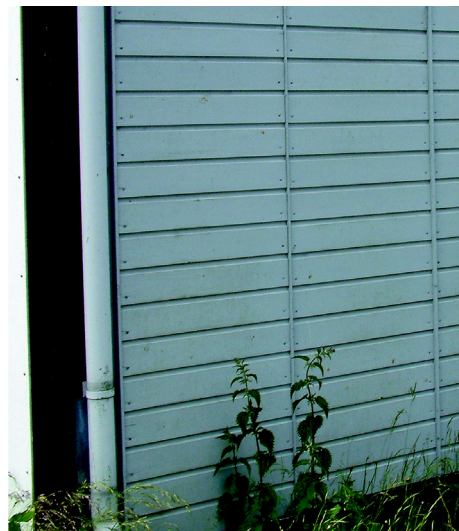
Figure 14 Section of north façade of test building, June 2009. Element 8 is to the left, next to the drainpipe. Algae are not visible on the cladding.
