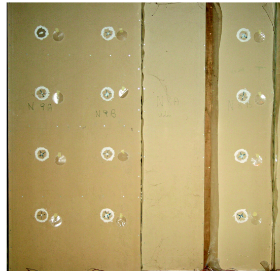
Figure 6 Elements with restored inner cladding after removing four pieces of vapor barrier.
