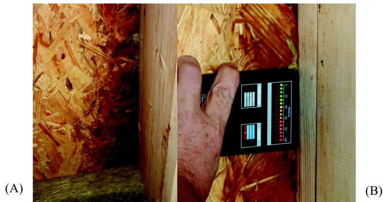
Figure 11 Element 8 facing north (horizontal weatherboard, nonventilated cavity, oriented strand board as wind barrier). (A) Wet part of the wind barrier seen from inside and (B) display on the handheld moisture meter indicating critical moisture content (i.e., all indicator lamps are on, including the red ones).
