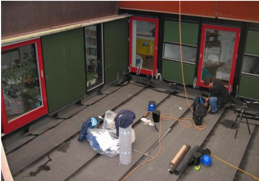
Figure 9: The membrane is installed in a roof terrace after replacing the two facades to create higher up stands.
