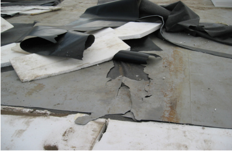
Figure 7: The loss of plasticizers was critical because it caused the membrane to shrink and become brittle.
