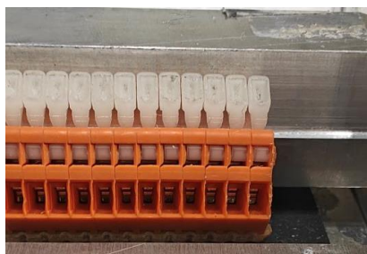
Figure 3. Close-up of the junctions in the compensation box.
