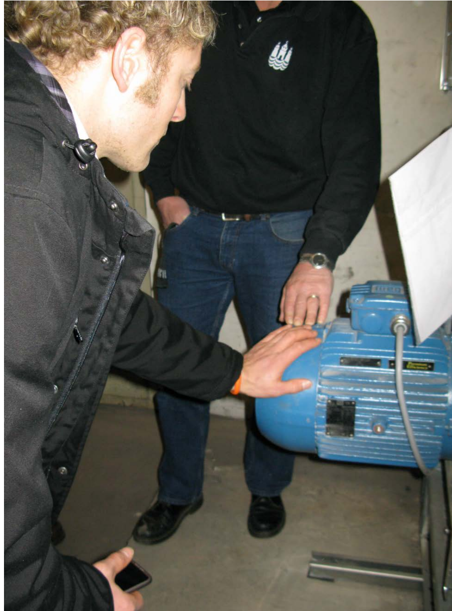
Figure 76. Circulation pumps are replaced mostly by low-energy models, which also facilitate and interface to the intranet. Photo: (Peter Vogelius).
