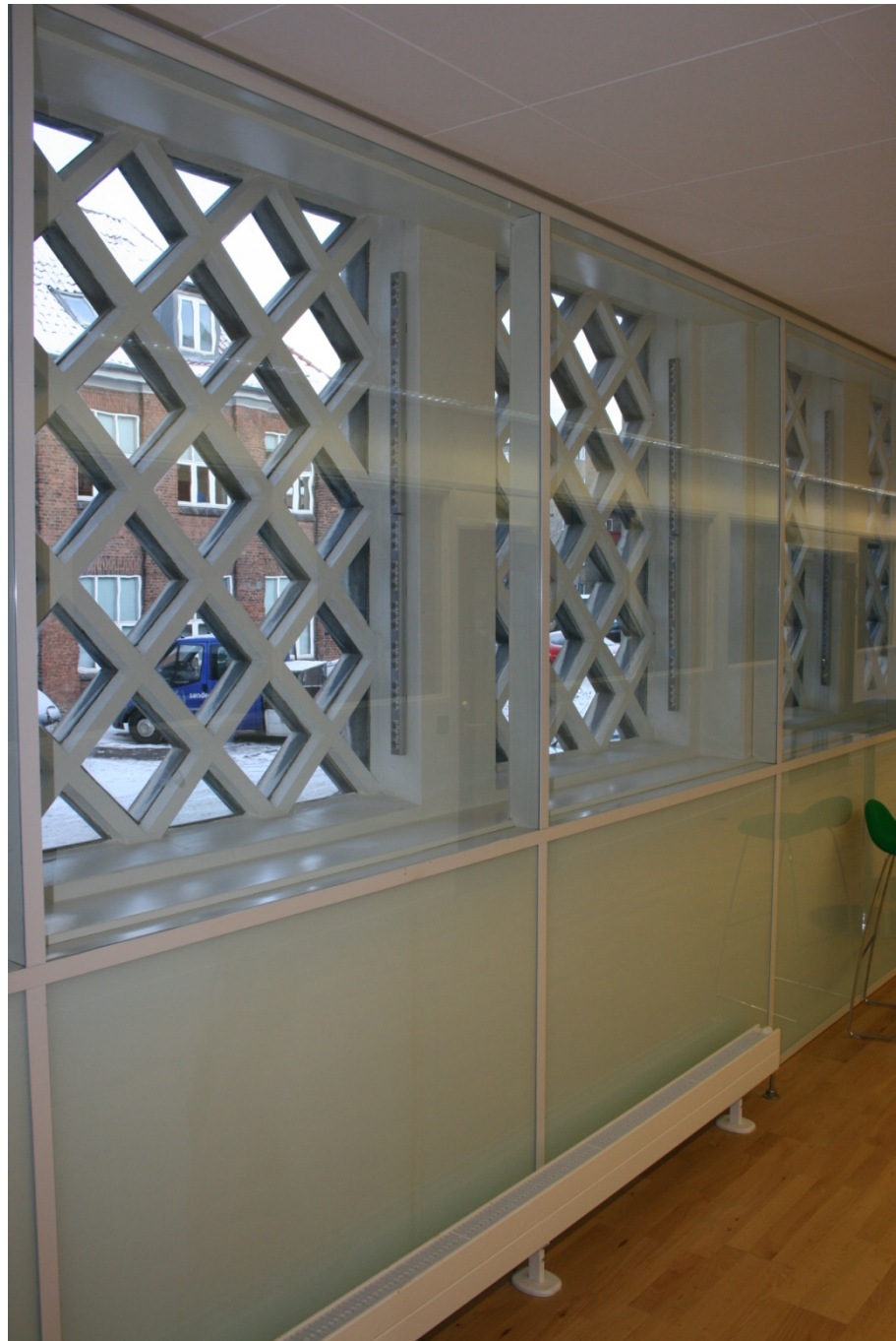
Figure 70. A solution was chosen where the whole facade was placed behind a “glass wall” (from the inside) as the very special windows could not be renovated in ordinary ways. Photo: (Kim Haugbølle).
