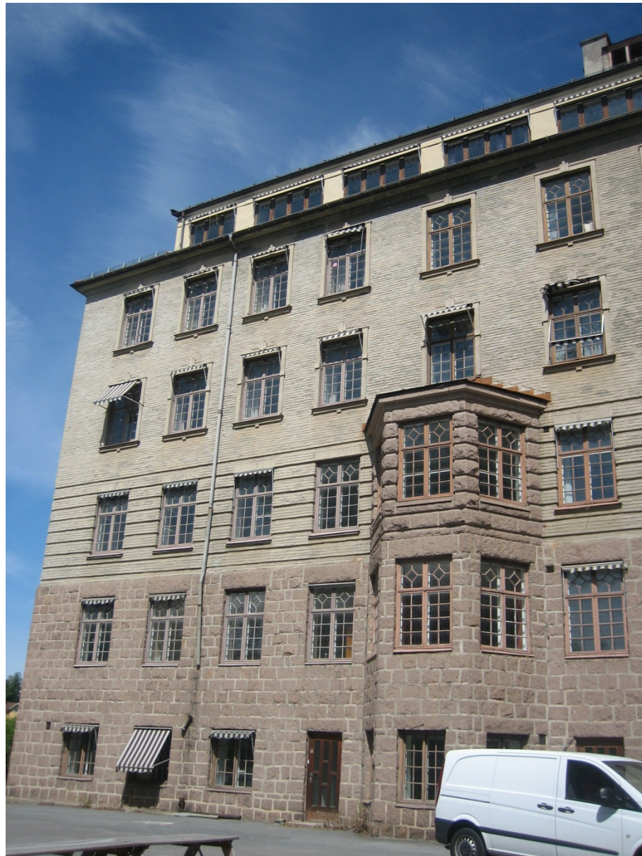
Figure 100. Outer wall façade. There is a clear distinction between the stone wall and the brick wall. Photo: (Anders-Johan Almås).
