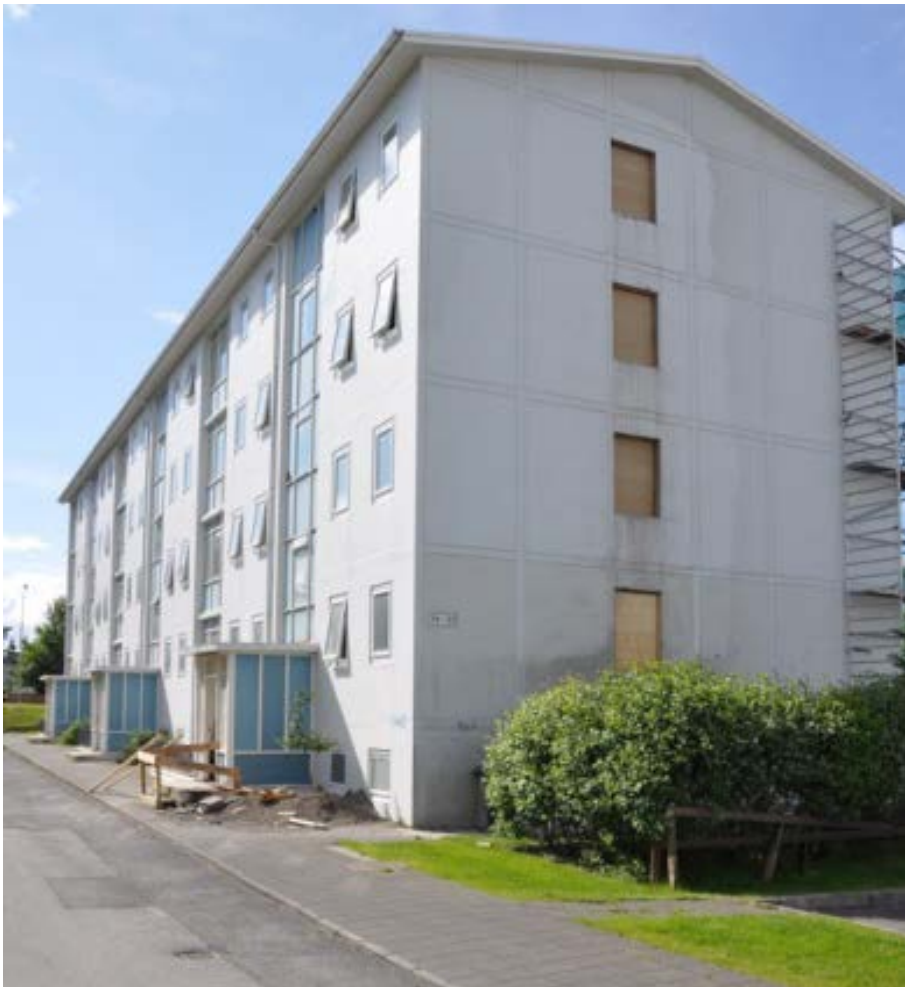
Figure 108. North view. New window openings have been cut out on the gable wall (during refurbishment). Photo: (Björn Marteinsson).
