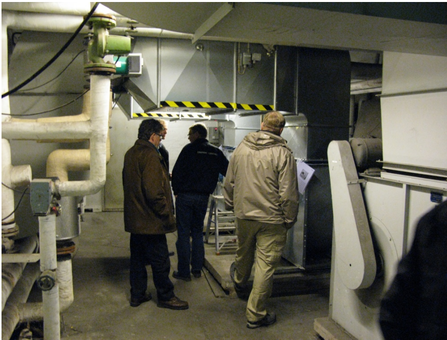
Figure 75. The old heating system is still working, but is part by part being renewed. Photo: (Peter Vogelius).
