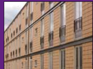
Multi-storey property after a façade renovation with an improved insulation and a new rain shield. Photo: Henrik Tommerup
