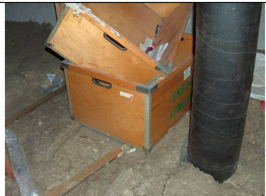
Dis-placed and compressed roof insulation.
