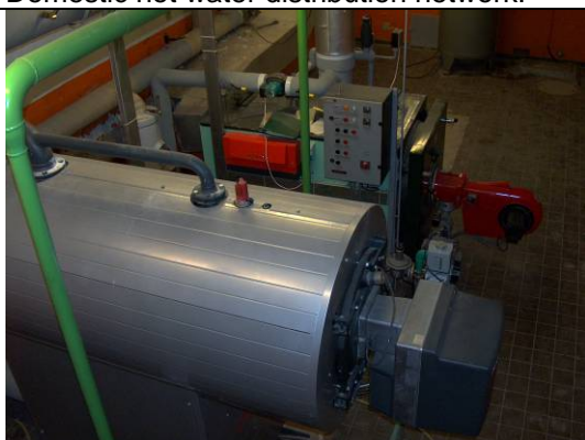
Boilers, condensing and traditional.
