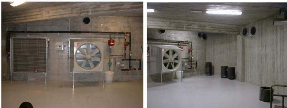
Figure 4.13. The air distribution room, showing the preheat unit (left) and fan, as well as the plastic subterranean ducts leading to the various rooms (Schild 2002a).
