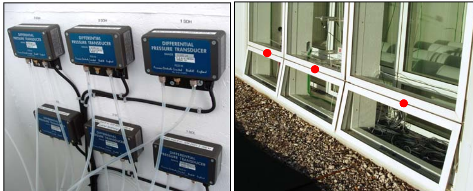
Figure 39. Pressure transducers Furness Controls Ltd. FC044 (left). Location of the pressure measurements at the window surfaces, SOL-openings (right).
