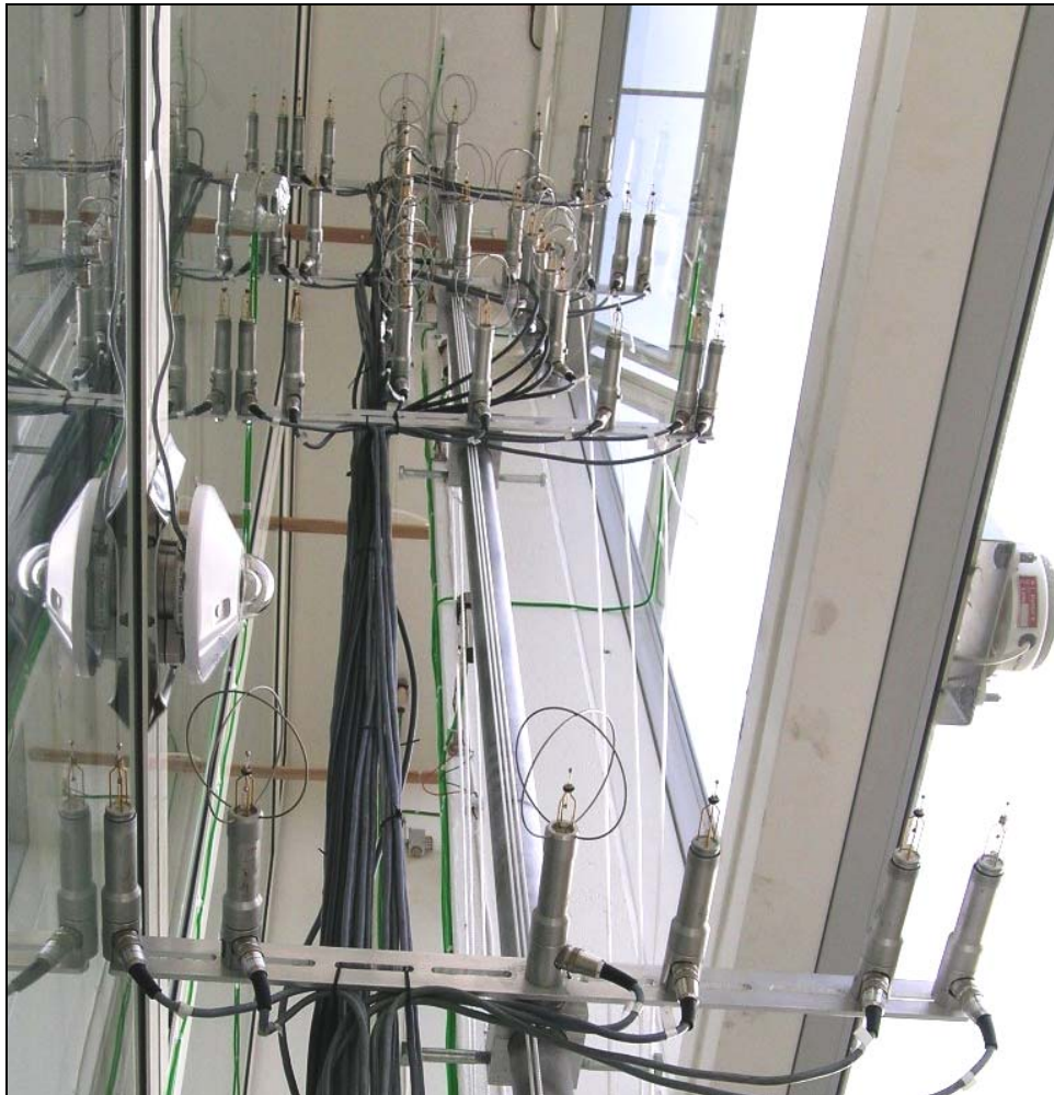
Figure 36. View to the final positioning of anemometers in the cavity (view from the bottom of DSF).
