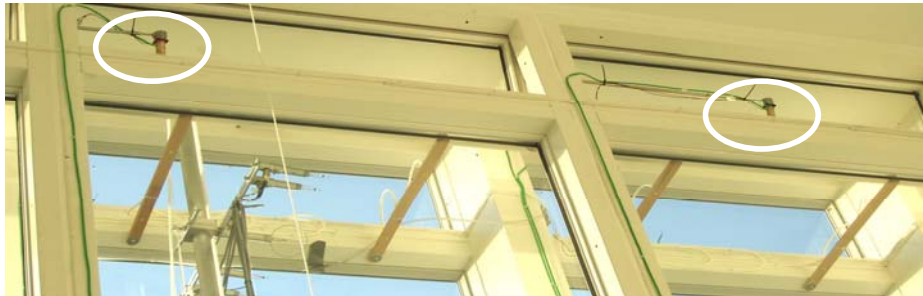
Figure 34. Measurement of outlet air temperature from the DSF.
