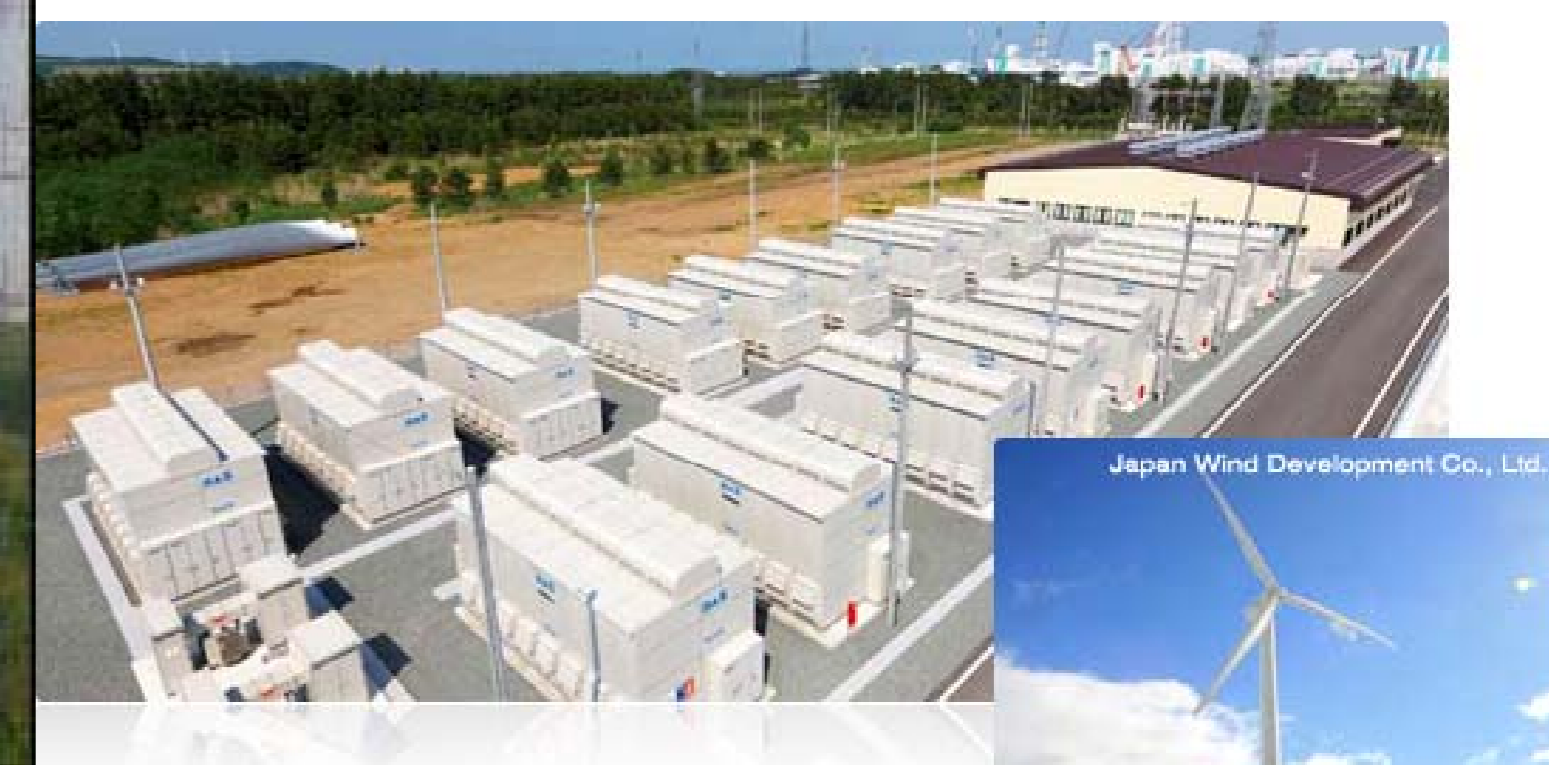
34MW NAS storage, Japan
