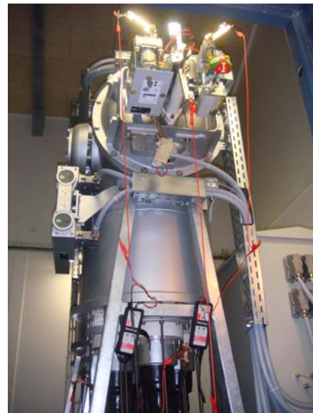
Fig. 10 Measurements on a GIS connected end of the 150 kV land cable
