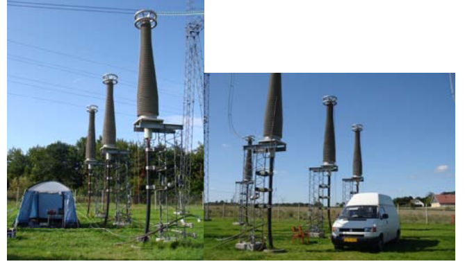
Fig. 5 Field test facilities at each cable end of the 400 kV cable system
