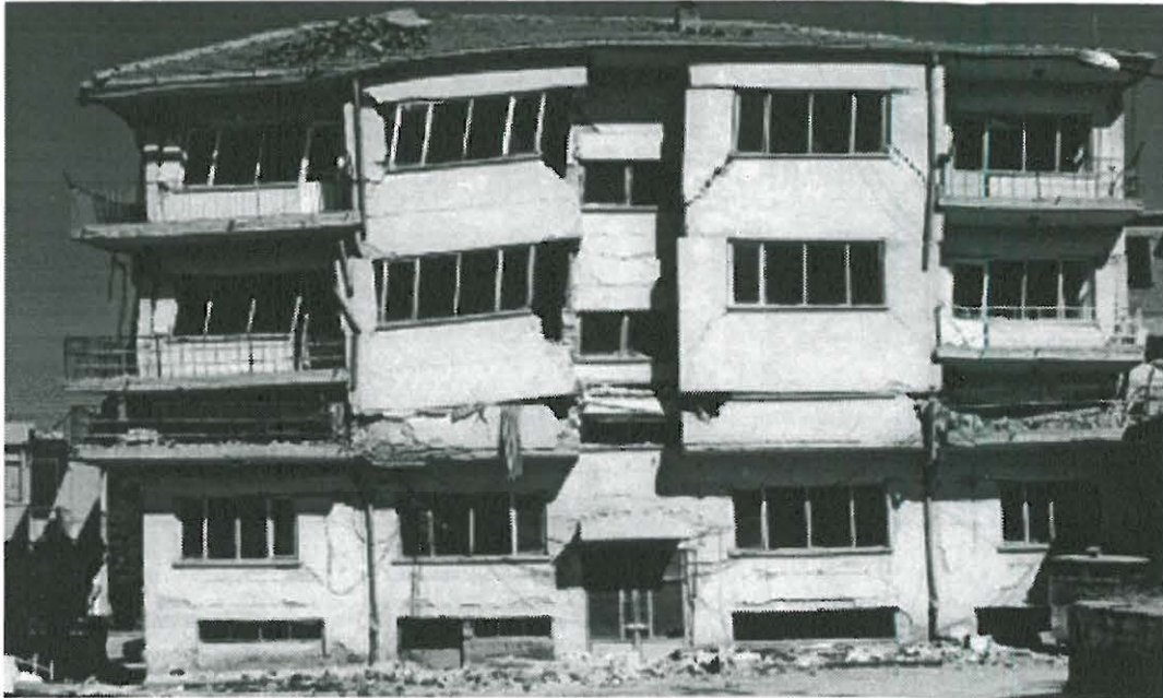
Figure 1.1: Collapse of an intermedia floor due to the October 1995 Earthquake, Dinar, Turkey.
