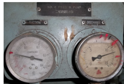
Fig. 2. Pressure measurement of auxiliary boiler feed water pumps on a ship in port before improvement
