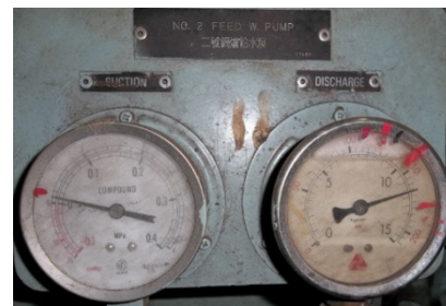
Fig. 2. Pressure measurement of auxiliary boiler feed water pumps on a ship in port before improvement
