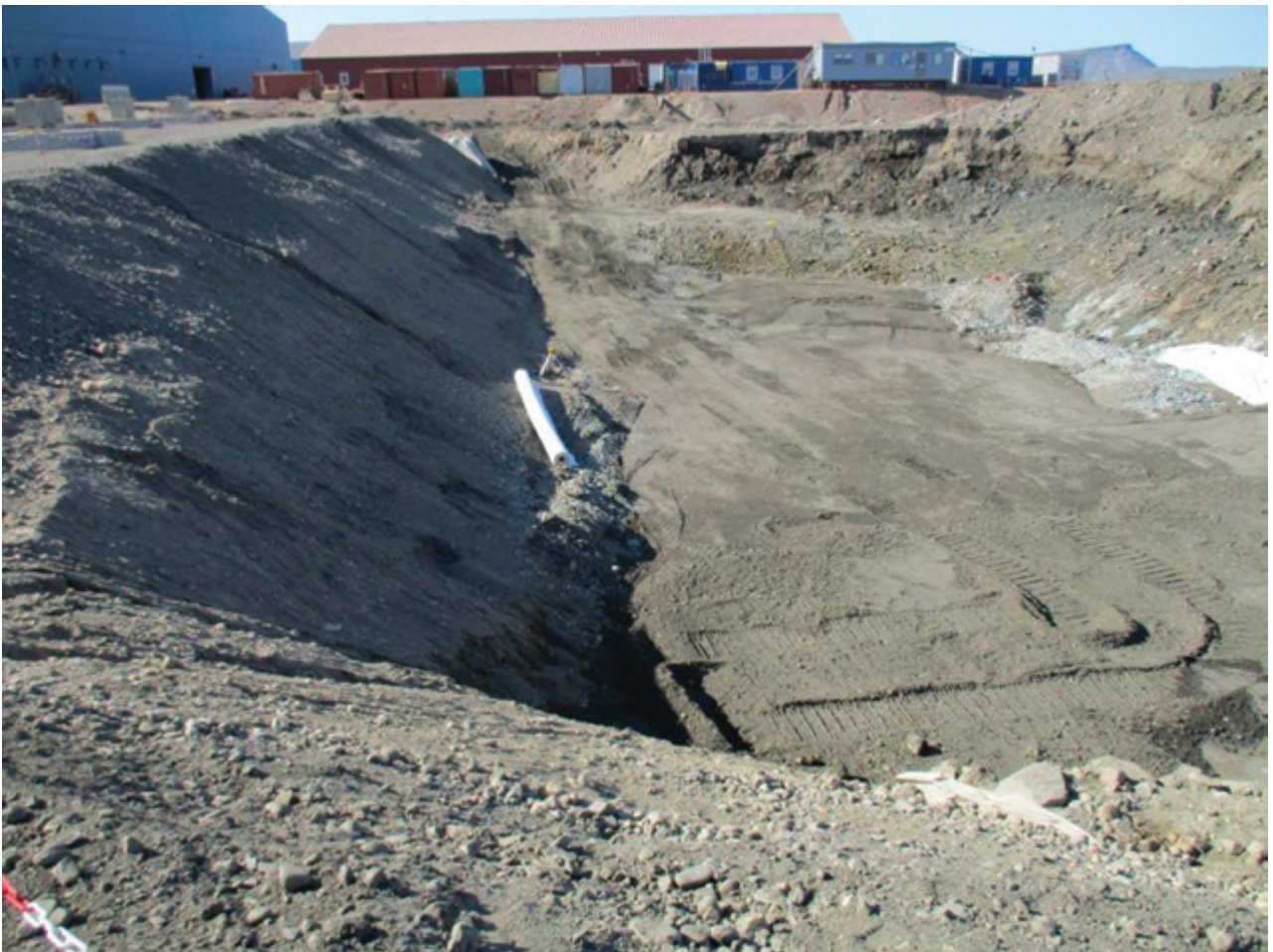
Figure 10.19 Over-excavation for construction of slab-on-grade structure, Thule Air Base (photo by Kevin Bjella).
