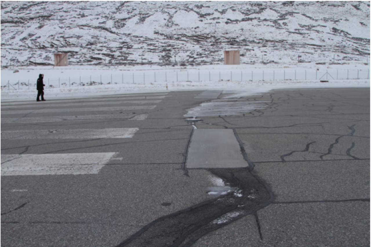
Figure 10.13 New repairs of pavement cracking and settlement at the west end of the Kangerlussuaq runway, November 2015 (photo by Thomas Ingeman-Nielsen).
