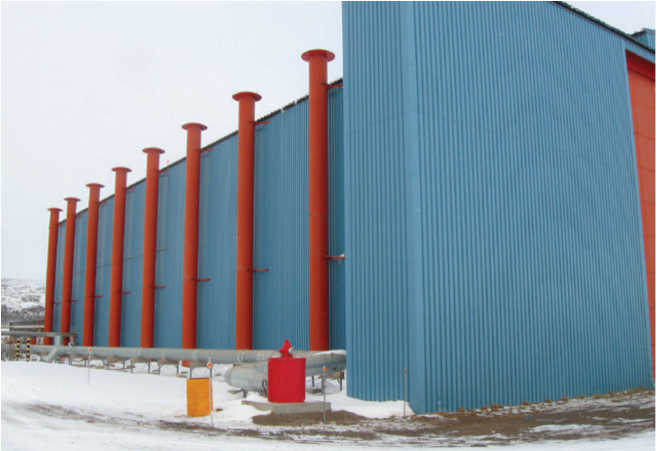
Figure 10.18 Aircraft hangar under-floor cooling plenums, Thule Air Base (photo by Kevin Bjella).
