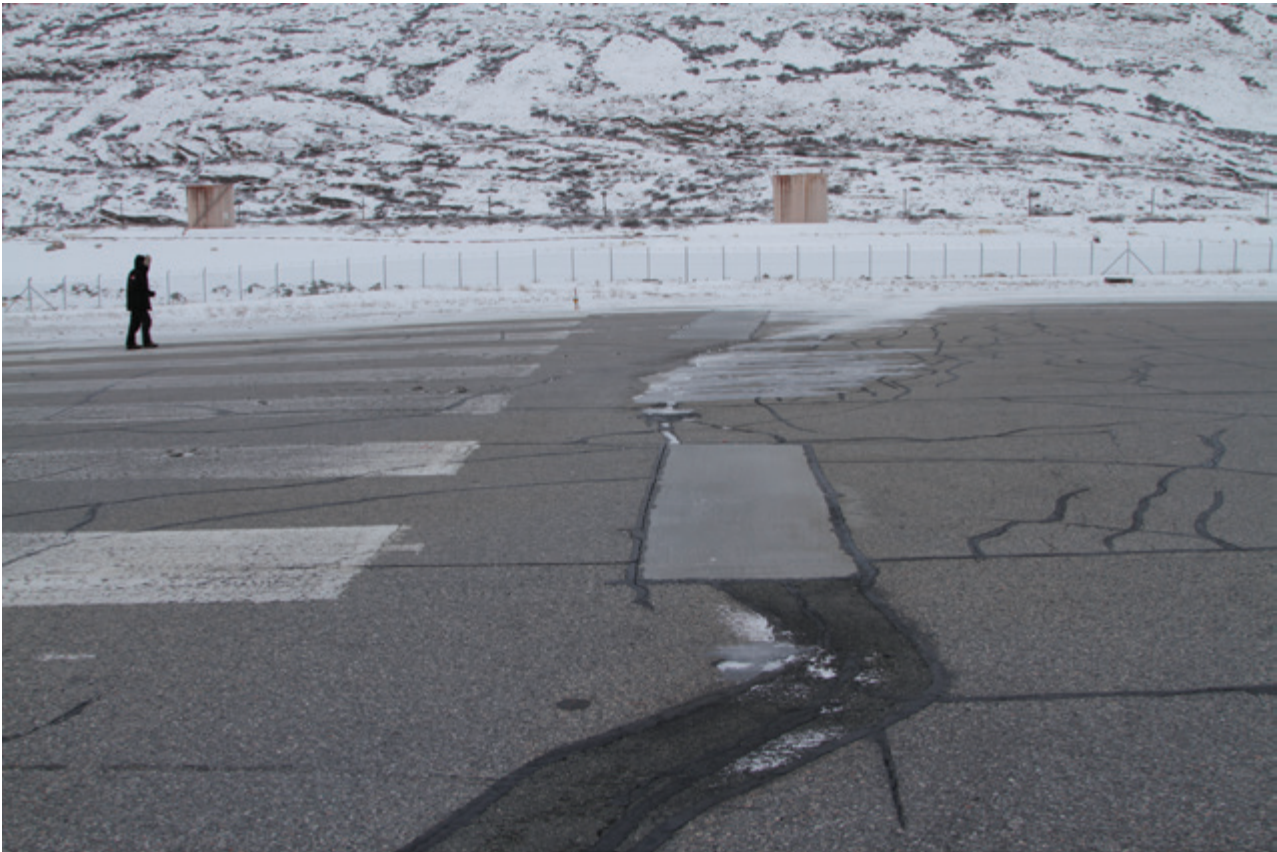
Figure 10.13 New repairs of pavement cracking and settlement at the west end of the Kangerlussuaq runway, November 2015 (photo by Thomas Ingeman-Nielsen).
