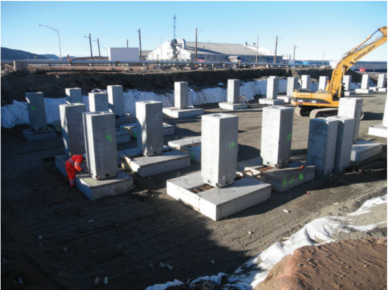
Figure 10.17 Excavation and placement of pier-and-footer style foundation for new dormitory, Thule Air Base (photo by Kevin Bjella).
