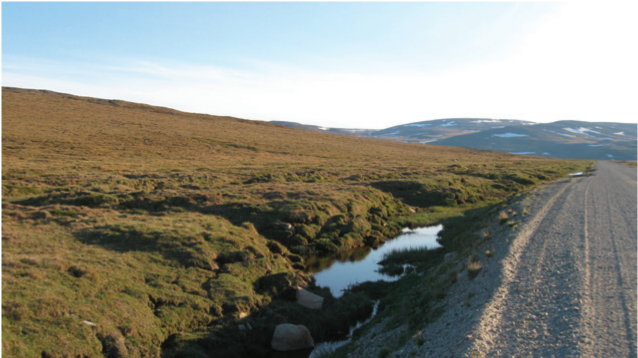
Figure 10.11 Water ponding in a depression created by thaw subsidence at the bottom of an embankment. This subsidence was facilitated by the thermal impact of a snow bank previously at the road's edge (photo by E. L'Hérault).
