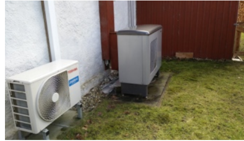
Fig 4: An air to water heat pump at one of the participating households.
