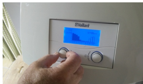
Fig 8: A householder viewing electricity consumption on the heat pump interface.
