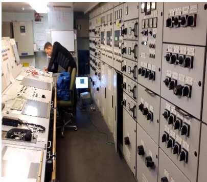
(b) Engine room
