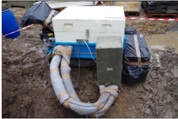
Fig. 1. Ongoing TRT at Langmarksvej. Inlet- and outlet pipes are insulated to prevent disturbances from ambient temperature conditions [2].
