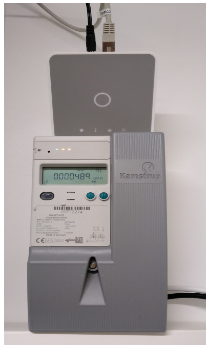
Figure 10. Kamstrup Smart meter.
