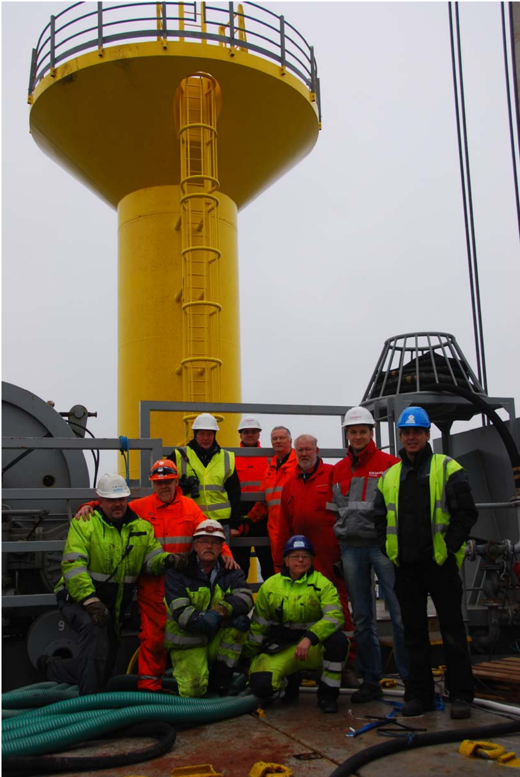
Successful installation of the first monopod bucket foundation offshore in Denmark First and second from the right: Lars Bo Ibsen and Christian LeBlanc
