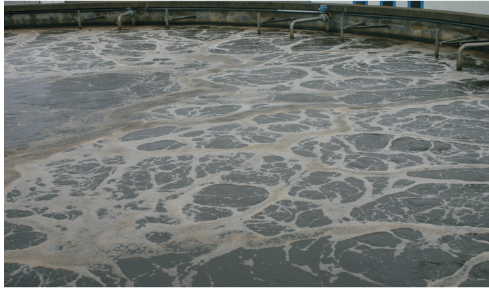
Figure 5.51 Picture showing part of the aeration tank at Frederikshavn Central WWTP during aeration.
