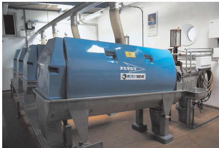
Figure 5.32 Drum screens at Hals Central Wastewater Treatment Plant.
