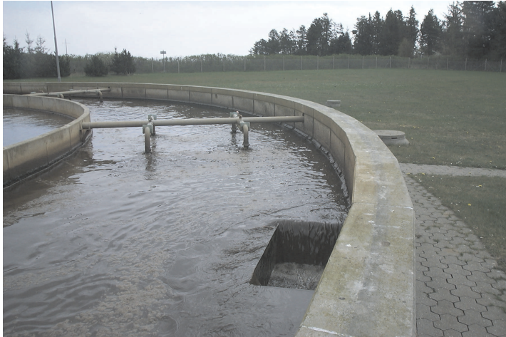
Figure 5.35 Outlet weir of the OCO-tank at Hals Central Wastewater Treatment Plant.
