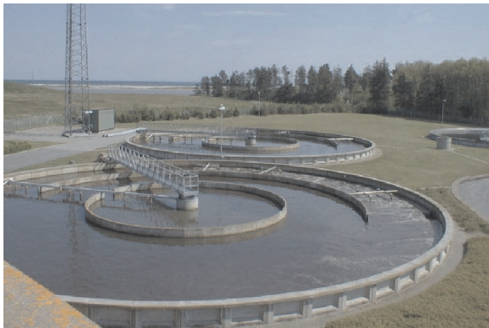
Figure 5.34 Overview of the to OCO biological removal tanks at Hals Central Wastewater Treatment Plant.
