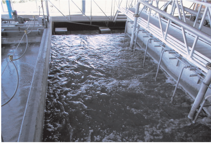
Figure 5.33 Sand and grease trap at Hals Central Wastewater Treatment Plant.
