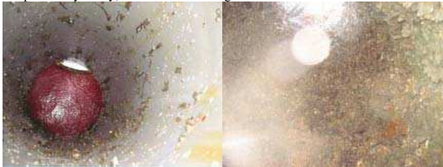
Fig. 13: The insides of two turbine draft tubes, on the left one painted with silicone paint, and on the right painting with conventional epoxy paint.
