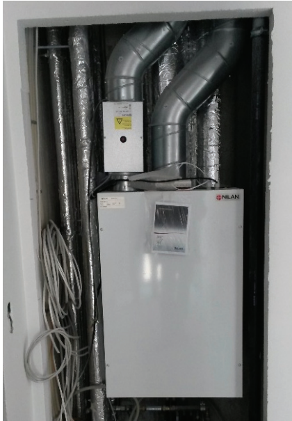
Figure 3.6: Decentral ventilation unit inside a cupboard in a flat.
