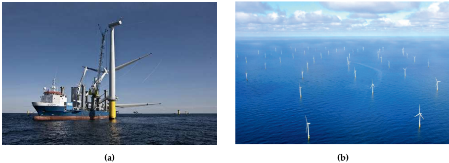
Fig. 1.1: (a) Installation of the first turbine at Horns Rev 2 (Kanter, 2009); (b) Horns Rev 2 offshore wind farm (Naturstyrelsen, 2014)
