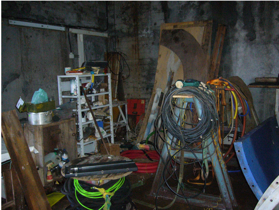
Figure 4.1 Pico turbine hall in 2007
