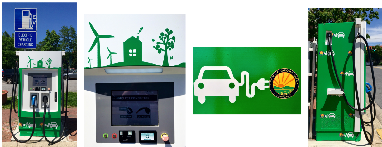
Figure 34 Cindy Herrera's design for EVSE in the city of Takoma Park, Maryland, USA ( https://takomaparkmd.gov/department/makeover-for-electric-vehicle-charging-stations/ )
