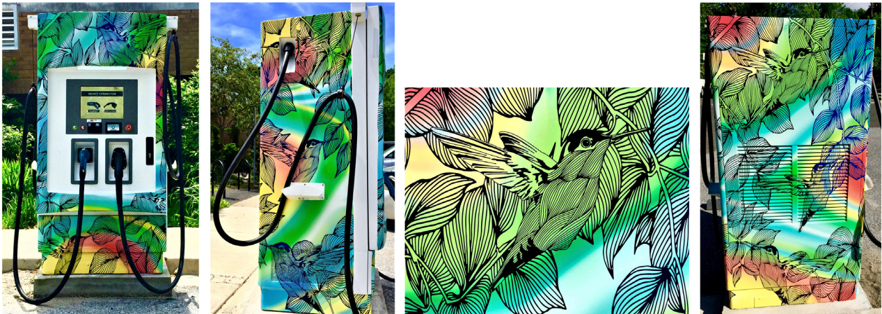
Figure 33 Jay Shogo's design for EVSE in the city of Takoma Park, Maryland, USA ( https://takomaparkmd.gov/department/makeover-for-electric-vehicle-charging-stations/ )
