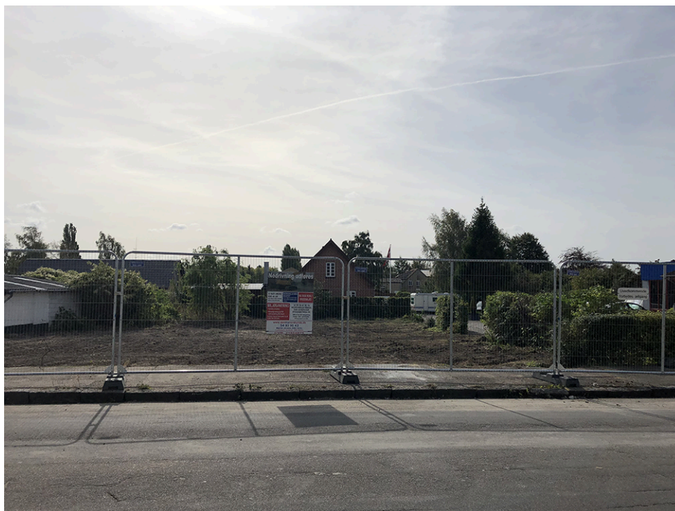
Plot after newly demolition of the house, Lolland municipality. Photo: Louise Ormstrup Vestergård.
