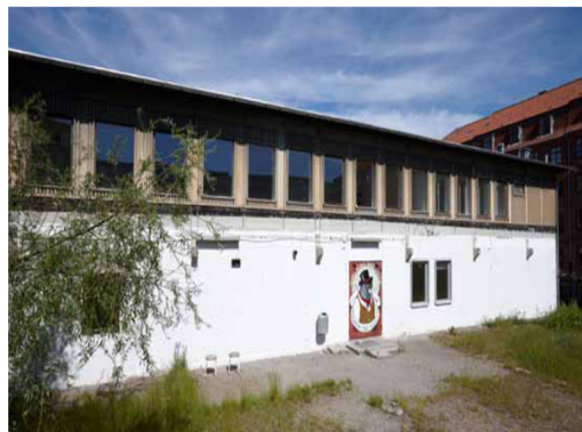
Figure 5. Façade facing the garden before renovation. The façade was originally the division between the office area (existing) and the factory area (which was torn down many years ago). The façade is not protected.
