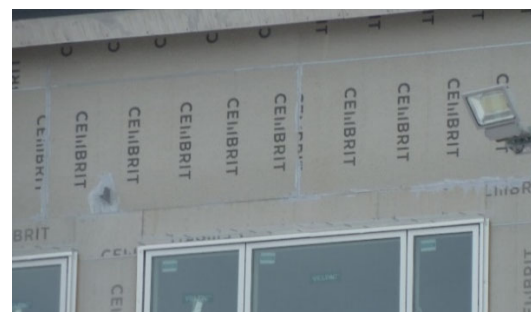
Figure 9. Facade before rain shield is installed showing the many joints that have to be sealed between fibre cement boards used as wind barrier.
