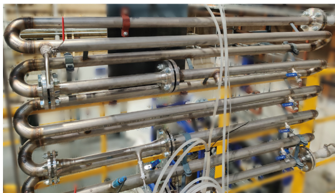
Fig. 2. In-line pre-treatment static flocculator. The flocculator consists of a set of 180° pipe bends and a metal coagulant is dosed at the inlet of the application and the dosing of the cationic polymer is performed after a total of 4x 180° pipe bends. The particle size distribution is measured at the outlet of the static flocculator.
