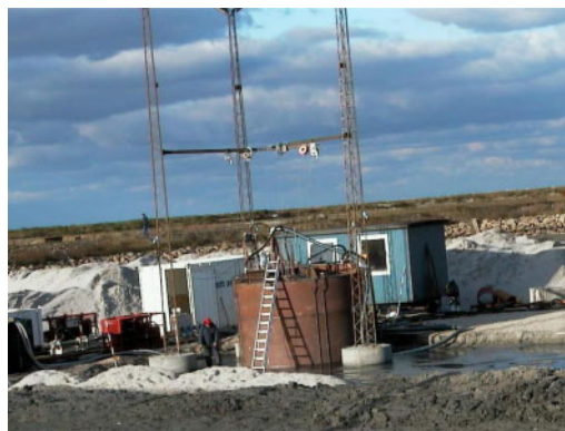
Figure 1. Installation tests on 4 \times 4 m buckets in a natural seabed at the test site in Frederikshavn, Denmark.
