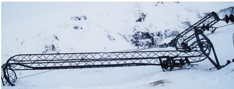
Fig. 1.4: A transmission tower after a heavy winter storm.
