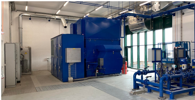
Fig. 1.13: The synchronous condenser at the wind farm substation in Suðuroy.
