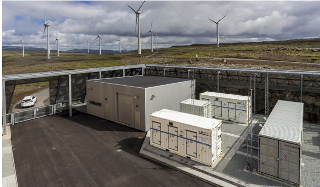
Fig. 1.11: The BESS located at the wind farm Húsahagi.
