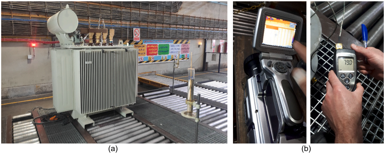
Fig. 15. (a) The studied 500 kVA DT during TRT in the HV laboratory, (b) thermography measurement of 500 kVA DT during TRT.
